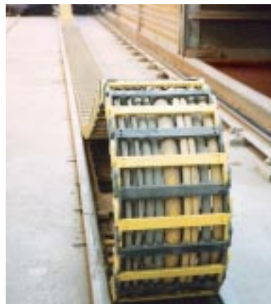
E4 in a pre-cast concrete plant with dust and concrete sediment
