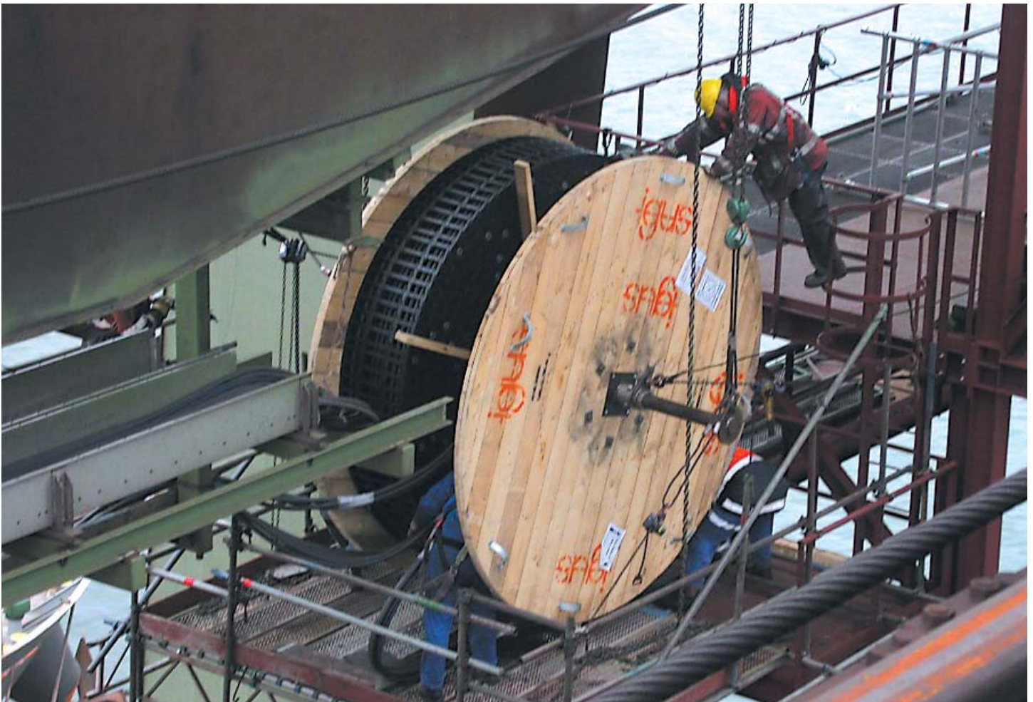
ReadyChain ® installation on a bulkhandling crane. ReadyChain ® system, including cable carriers and cables, weighs more than two tons.
